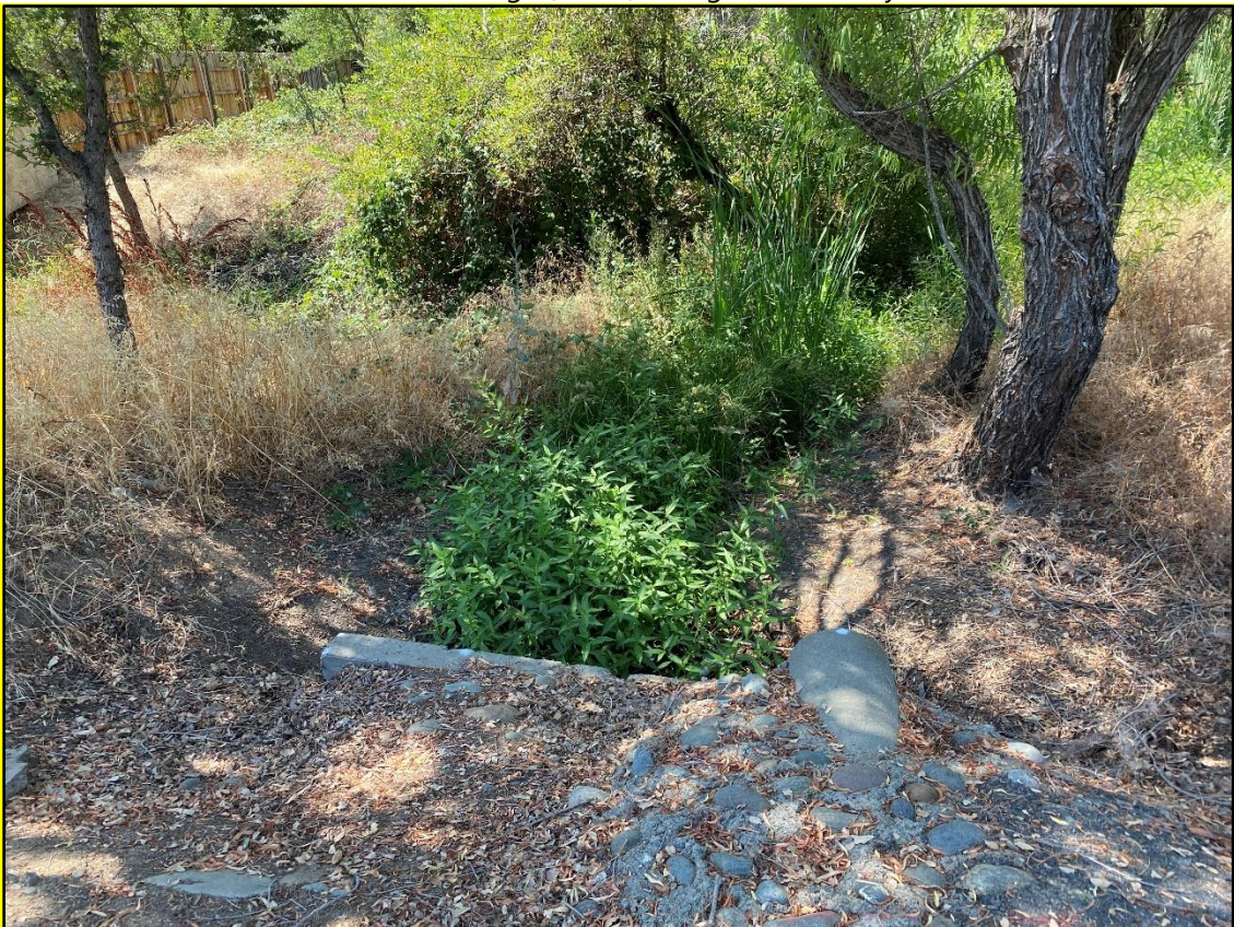
Intermittent drainage (IDR-2) upper reach, City storm drain outfall facing south, 23 July 2020
